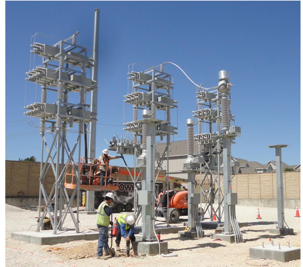
Seward Junction Substation
